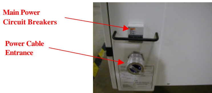
Figure 1.3 Circuit Breaker / Power Cable Entrance
